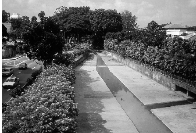
Figure 2.3 Canalized natural channel in concrete between Bukit Timah and Dunearn Roads in Singapore
